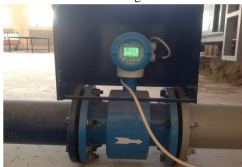
Fig. 2 Magnetic flow meter.
